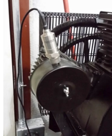
USB Digital Accelerometer on Air Compressor
