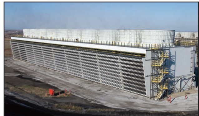
Photo Courtesy of Midwest Towers, Inc.
