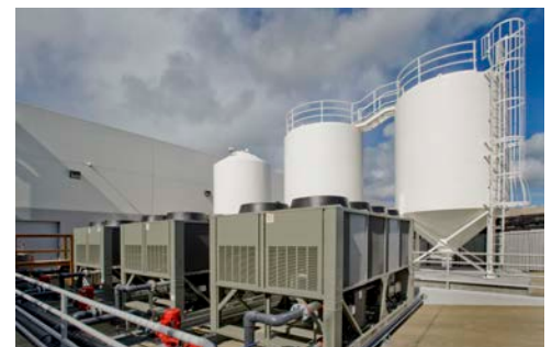
Air-cooled condensing unit
