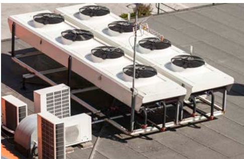
Air-cooled heat exchanger
