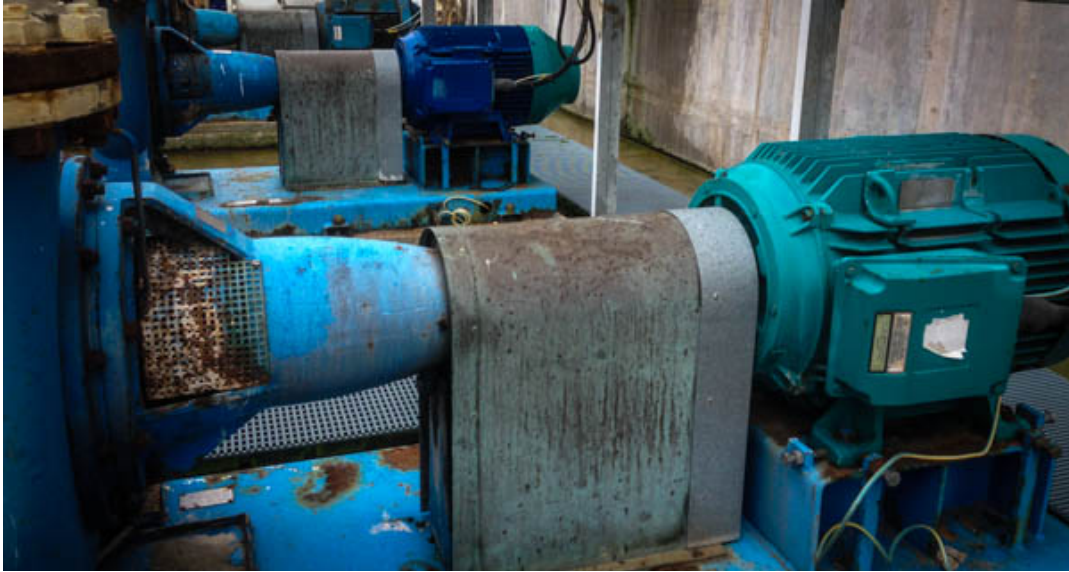
Figure 10 Cooling Water Pump
