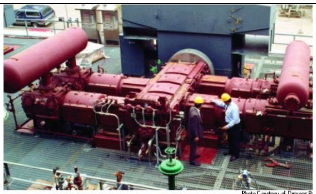
Figure 1(b) – Reciprocating Machine Vibration Monitoring
