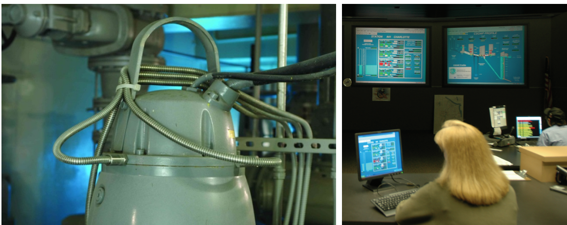
Figure 11: Permanently mounted IMI 4---20 mA output sensors on a vertical pump that are being continuously monitored by a PLC. (Photo courtesy of Monroe County Water Authority).
