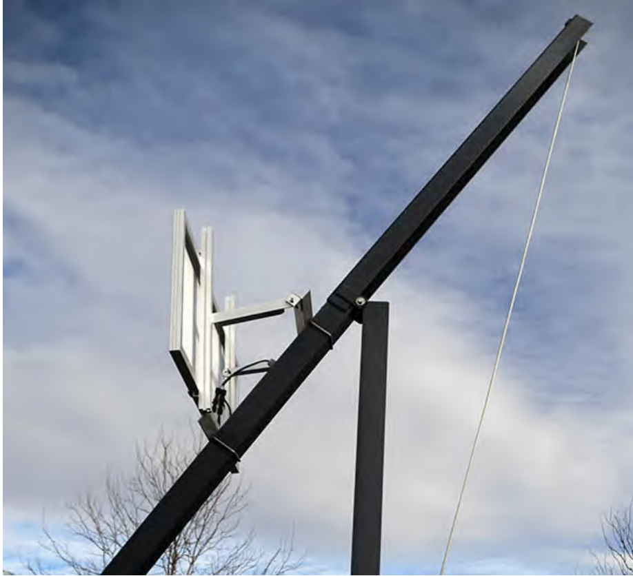
FIGURE 4-7 Solar Panel on Tip-Down Pole
